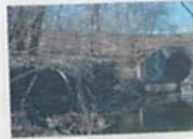
Eroded Stream Banks along Huron Parkway
